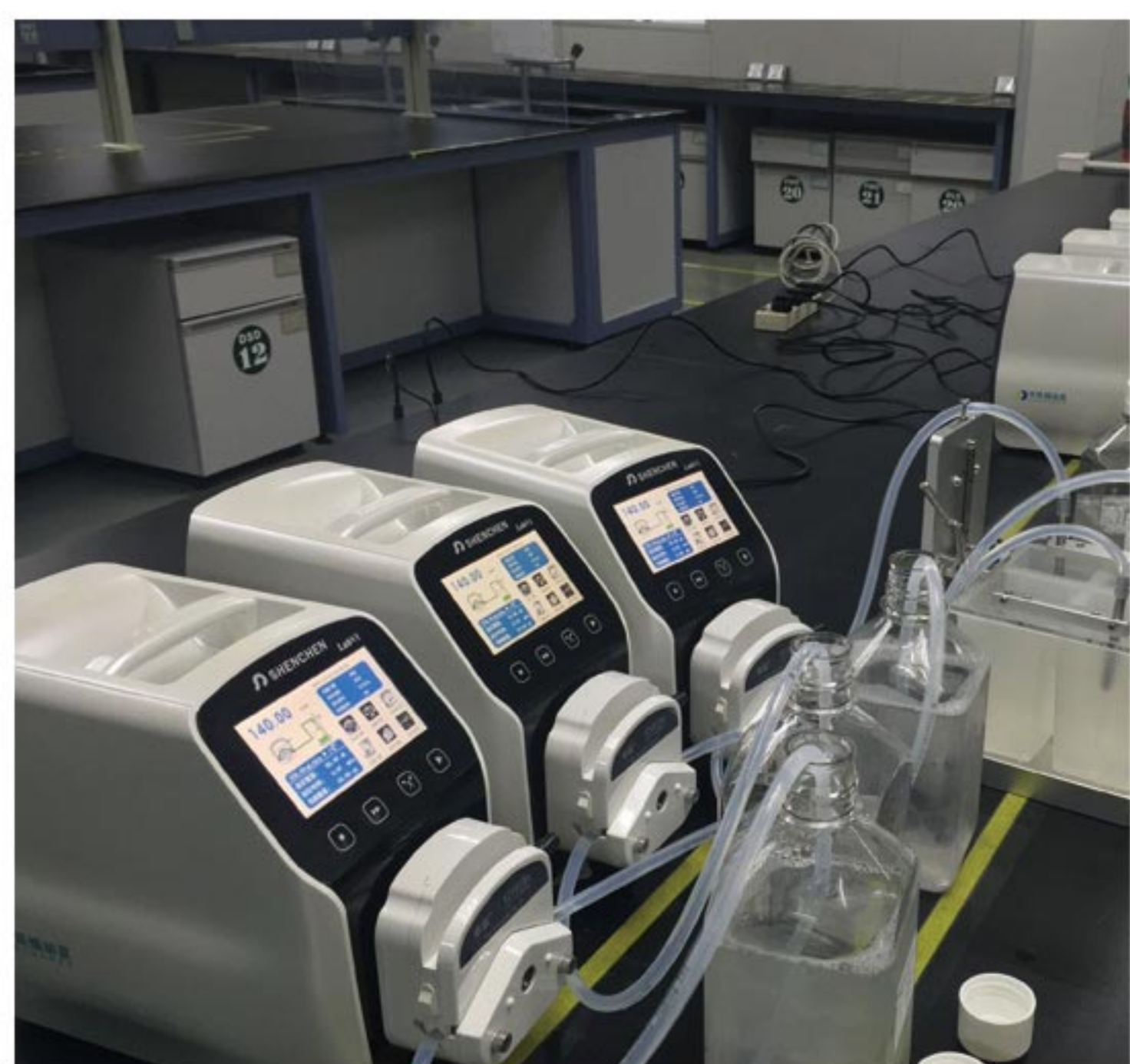
Laboratory chemical dosing
