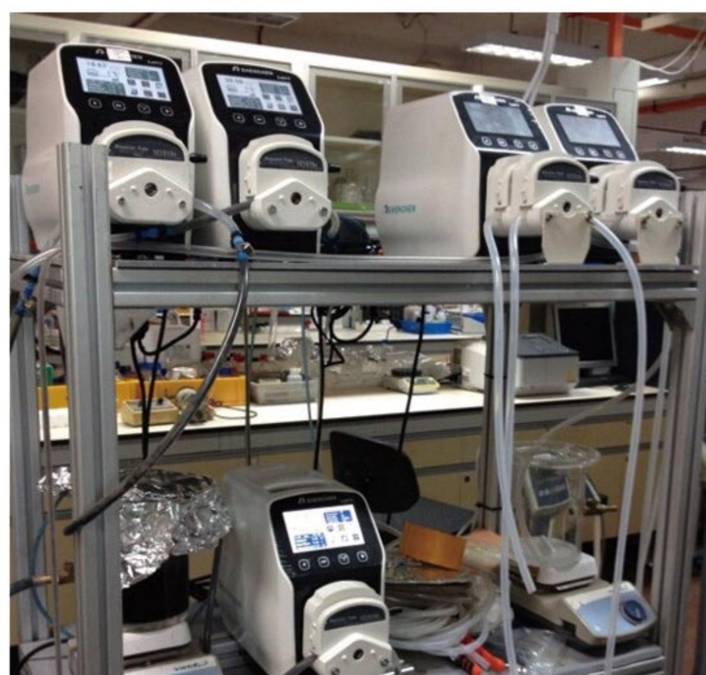
Waste water treatment
